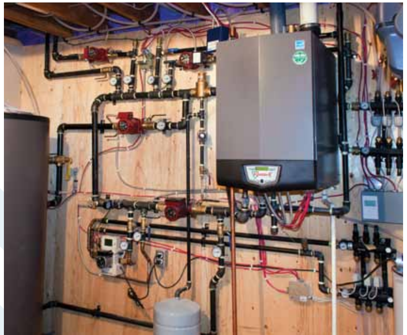
The Moes replaced all the electrical wiring and plumbing in the home to accommodate the latest technologies.
